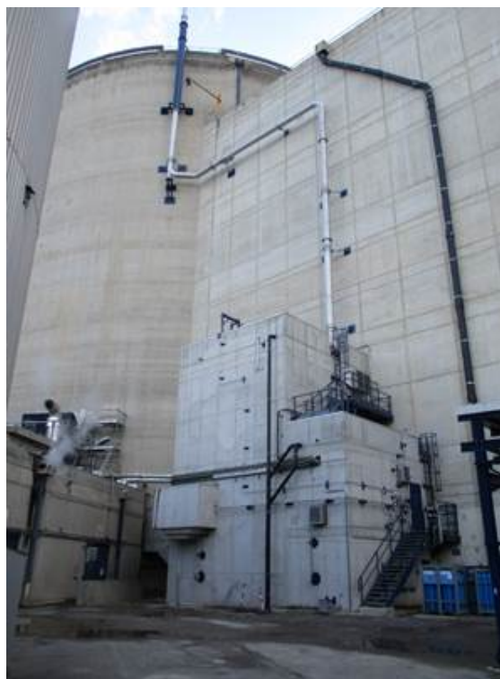
Figure 7 : Filtered containment venting systems of Tihange 3
