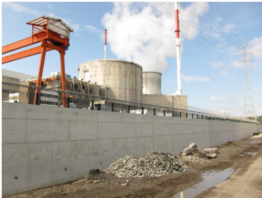
Figure 2 : Peripheral protection of the site of Tihange against beyond-design flooding realized in 2015
