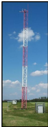
Figure 8. Illustration of a station installed on a 30 m mast around Belgian nuclear sites (MET 30 station) which measures wind speed and direction, pluviometry and sunshine.
