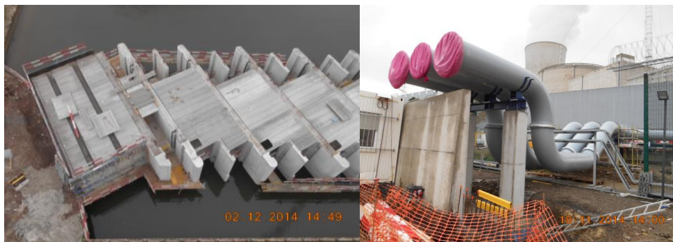
Figure 3: Construction of the water intakes (left) and the outlet pumping chambers (right) of Tihange 2
